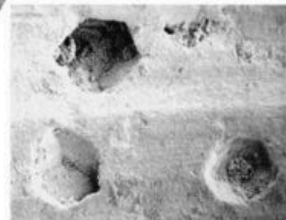
Holes arising from grit pop out
